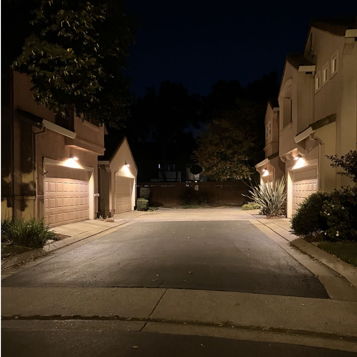
APTO 2200K full cutoff wall packs installed at Villa Palazzo in Sacramento, CA
