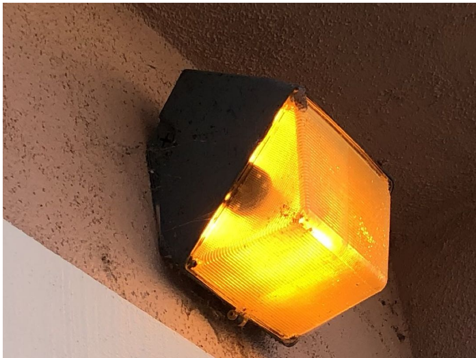
Before: 35-watt HPS wall pack, prismatic drop lens — a bare source in direct view.
