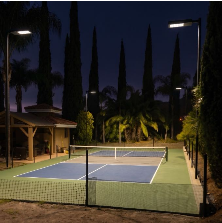
ASTAs illuminate tennis courts at a private residence in California.
