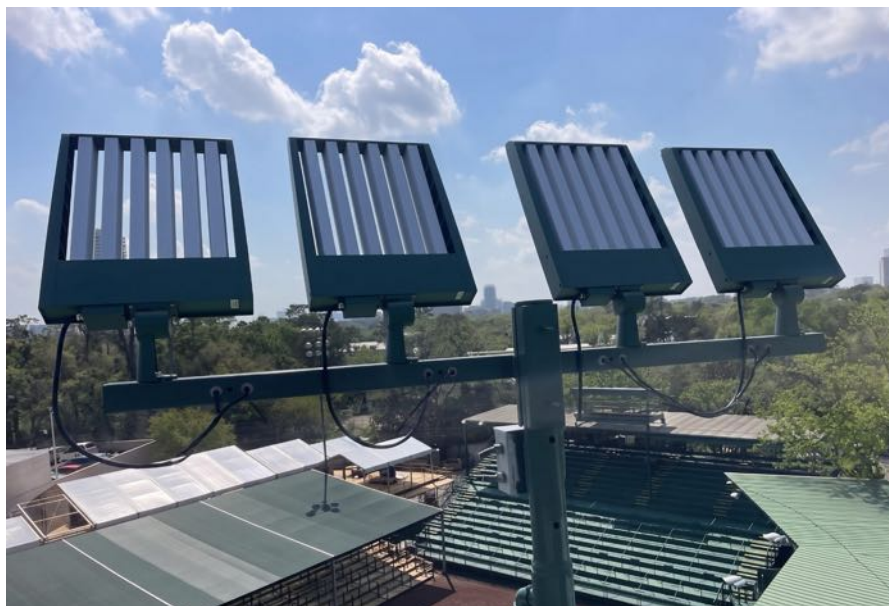
A four-luminaire cross-arm cluster over a clay stadium court, finished to match the venue.
